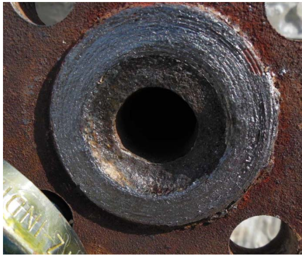
Figure 14. NPS 1" Class 150 SCH 160 Carbon steel flange corroded by HCl.
